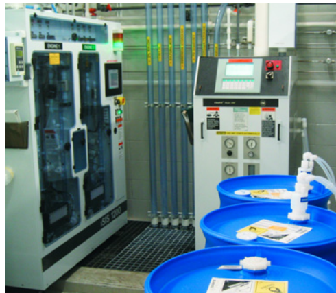
Entegris' chemical delivery solutions ensure against unsafe mixing and maintain chemical integrity. Photo courtesy of Cypress Semiconductor Corporation.
